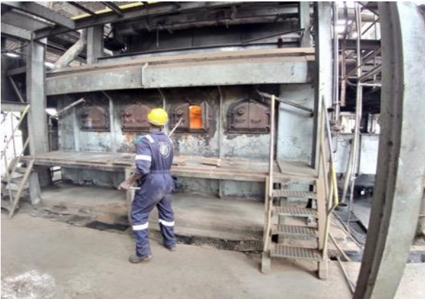
CHP boiler furnace (Francis Kemausuor)
