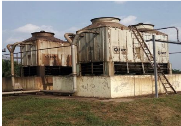
POME cooling towers (Evans Tenkorang, GOPDC)
