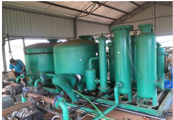
Gas purification and bottling plant (Hannes Muntingh)
