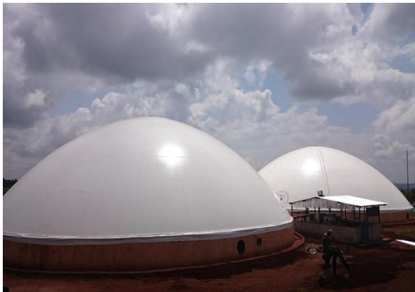
Twin digesters and gasholder control room (Hannes Muntingh)
