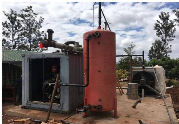
Exhaust heat exchanger, buffer tank and emergency cooler (Hannes Muntingh)
