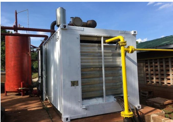
Containerised generator unit (Hannes Muntingh)
