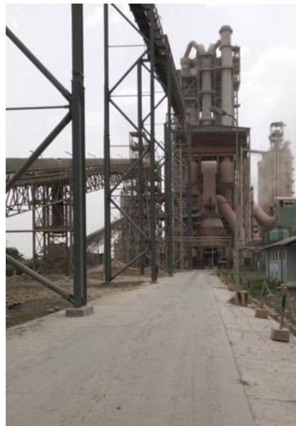
300 m inclined conveyor from AF plant to pre-calciner, Ewekoro II
